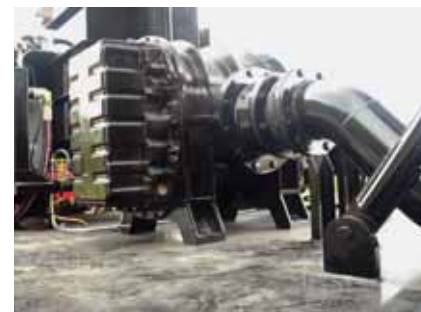
Aerzen Blower at the "heart" of the operation
