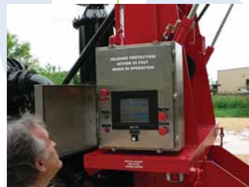
Mat Comardo at the control panel
